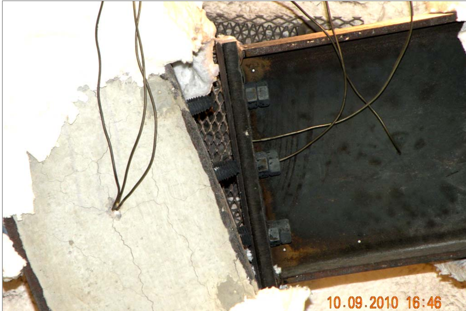
Failure mode: tensile failure of the bolts
