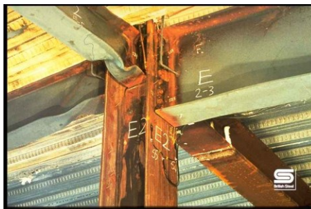
Figure 1. Shear buckling observed after one of the Cardington fire tests [2].
