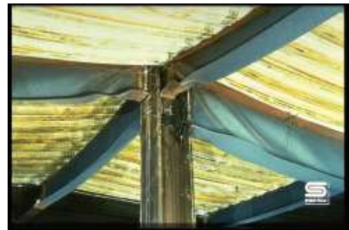
Fig. 1. Shear buckling and bottom-flange buckling in Cardington fire test [4]
