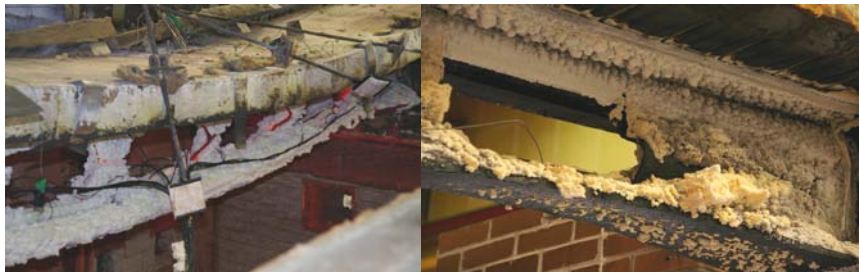
Figure 15. Web-post buckling failure mechanism.
