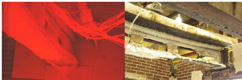
Figure 4. Intumescent on the bottom-flange fell off the beam near the support.
